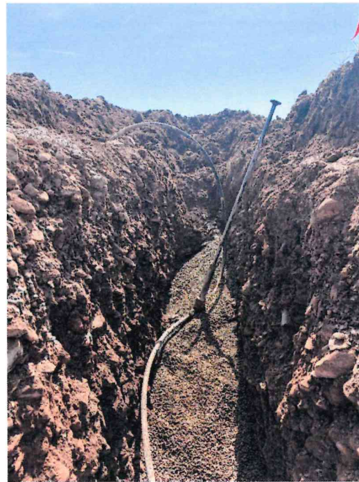
Water service and curb stop
