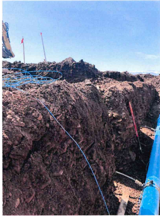
Water service tap and saddle
