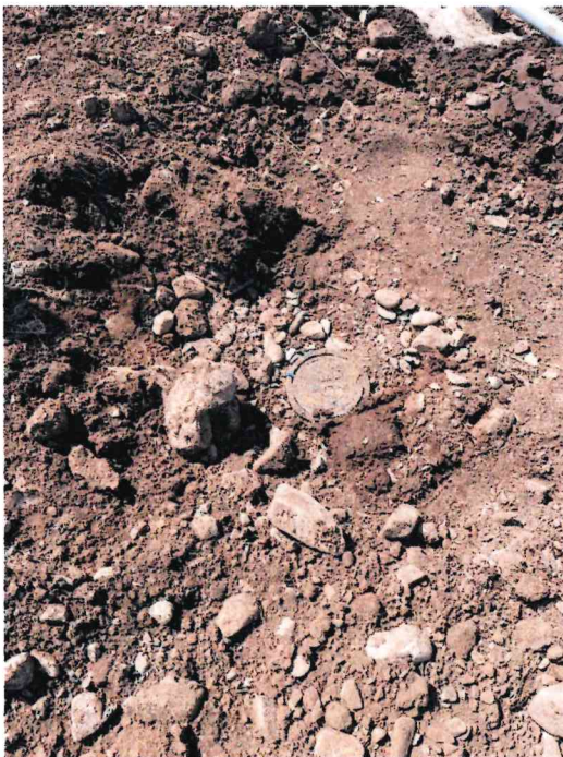
Water valve riser cap
