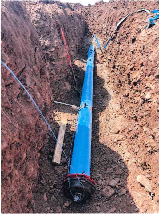
Water service, saddle, and cap
